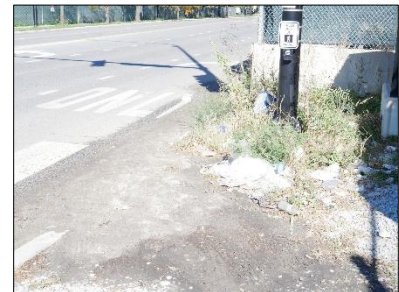
No Accessible Route Provided
