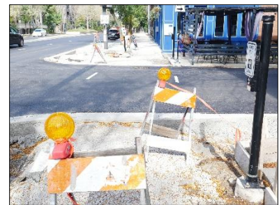
APS Device Obstructed by Construction Material
