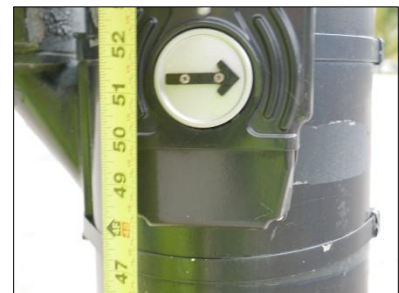
APS Pushbutton too High
