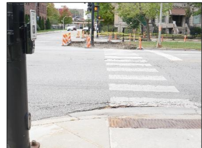
APS Pushbutton too High
