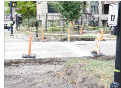
No Accessible Route to APS Device
