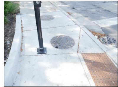
Accessible Route < 36" in Width
