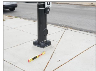
Excessive Slope on Route
