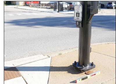
Excessive Slope on Route
